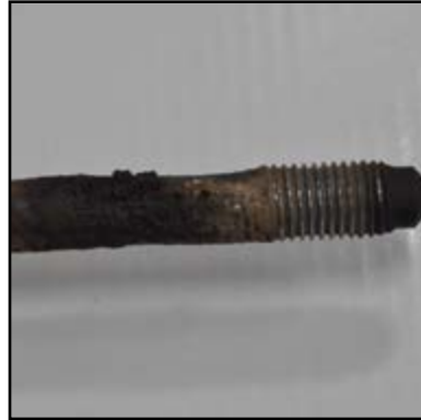
Rusted away and weakened bolts and fasteners
